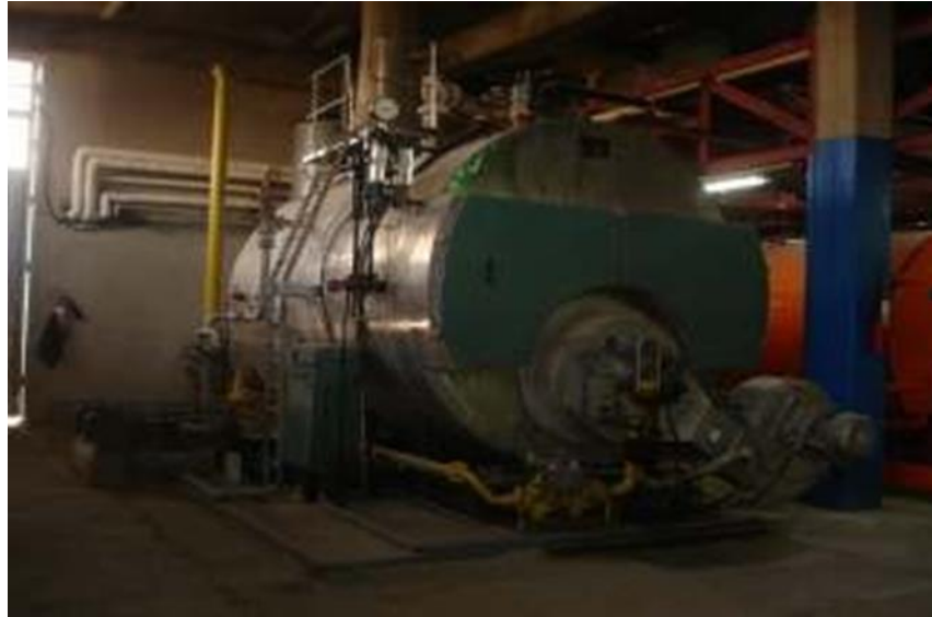
Figure 1-3 Boiler No. 1 with burner
