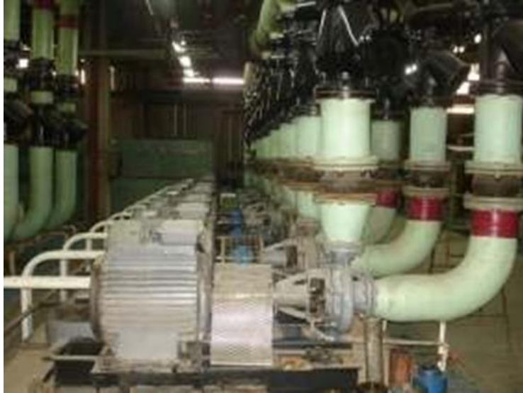
Figure 1-4: water circulation pumps
